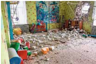
High tensions: A view of the kindergarten interior after the alleged shelling by separatist forces in Luhansk, Ukraine. *AP
